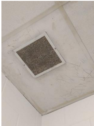
Figure 1. Stained, darkened ceiling tiles surrounding bathroom ventilation units
