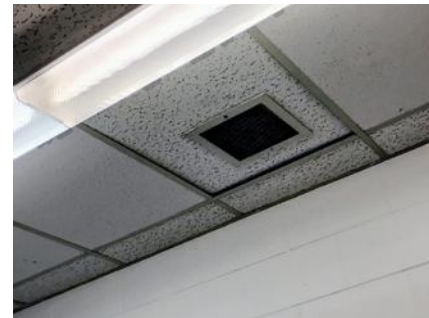
Figure 2. Broken/displaced ceiling tiles reveal dangerous student practices of hiding substance use
