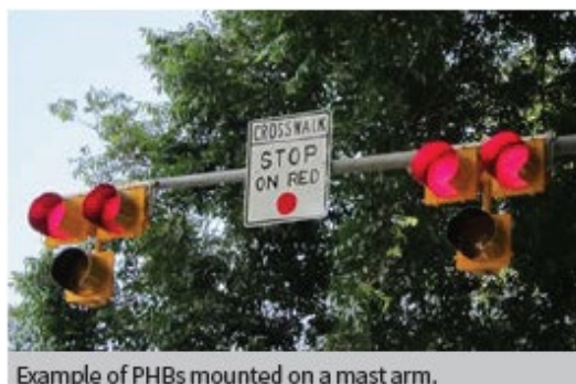
Example of PHBs mounted on a mast arm.
